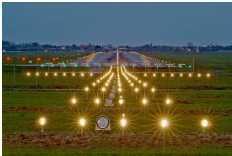
Airport Runway & Approach Lighting
